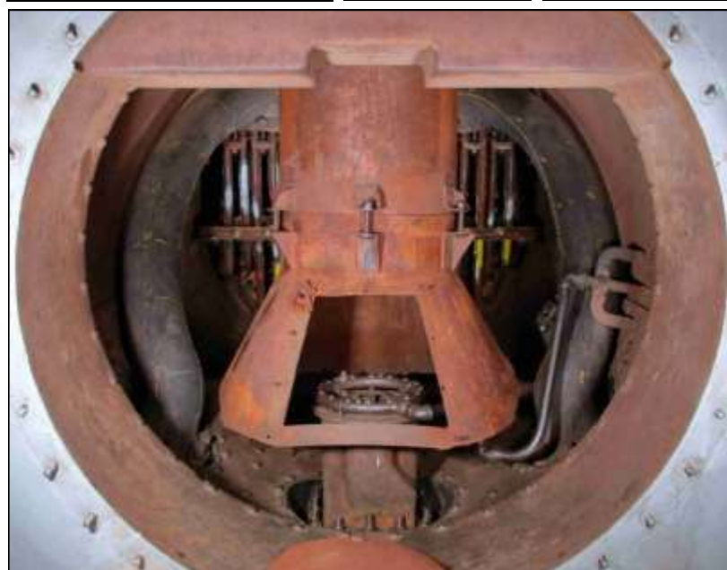
One Last Look Inside: From now on, the top of the stack will be easily seen whether extended or not, but this is a last peek inside the smokebox. Ron Taylor shot this picture before the front door was closed and bolted shut.
