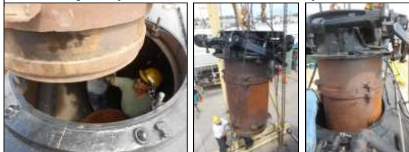
Below: The reassembled and tested stack is hoisted above the locomotive, lowered through the top of the smokebox and inserted into the petticoat.
