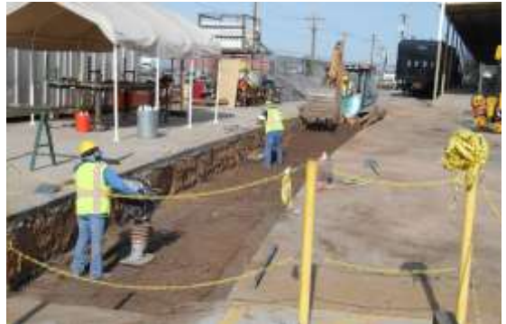
Dirt Work: Universal Constructors excavating and compacting the west (concreted) portion of the spur.
