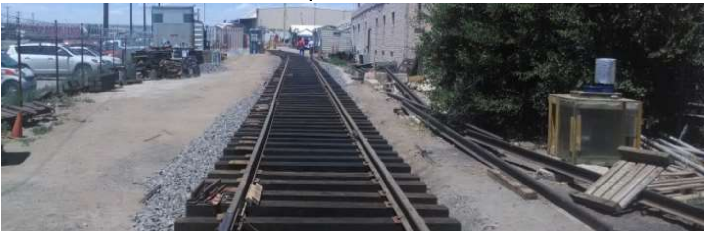
The 2926 restoration site June 2014: In this photo taken from 8th St NW looking west to the GSA warehouse the new spur is almost finished. The locomotive and tender were parked adjacent to the GSA warehouse (top Center) loading dock during track construction.
